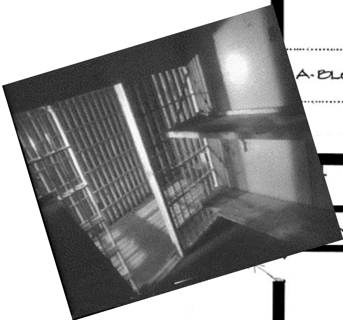
Photo showing DPD cell with solid walls between this cell and the other two in the area..
